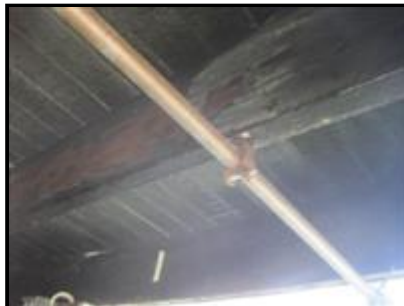
C. Picture 1 Fire damaged joists in NE corner
