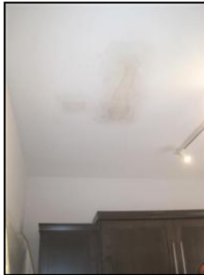
C. Picture 1 Wet area on bedroom ceiling
