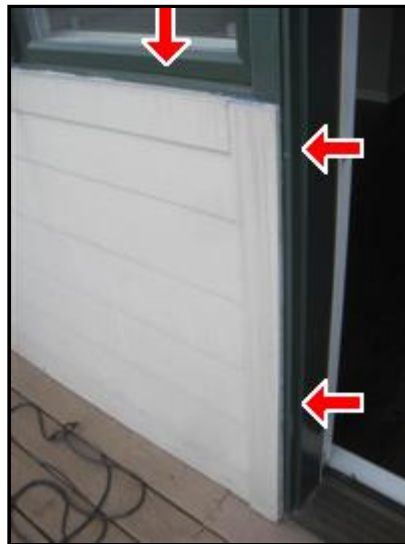
C. Picture 3 Recently caulked siding near door
