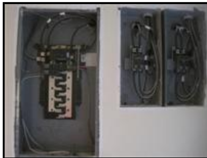
C. Picture 1 Public panel on left, 2 shut-off panels on right
